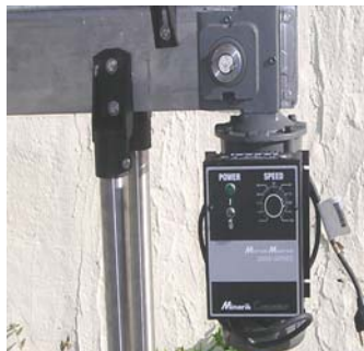
Variable speed drive (SPEED CONTROLLER)
